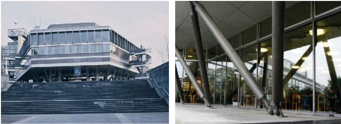
Figure 1.8: Retrofit intervention with 3Dp steel exoskeleton of the Hörsaalgebäude Physik building in Zurich [11].
