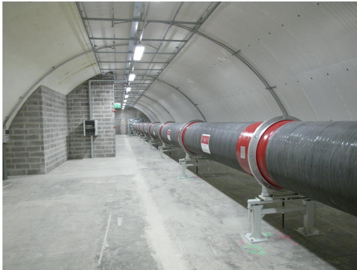
Figure 3.2: The Long Pipe at CICLoPE, 111.5m long and with a circular cross-section with a diameter of 0.9m.
