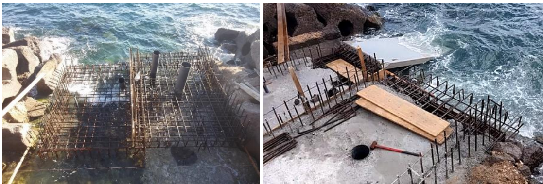
Figure 58. Construction of the bottom slab and positioning of the prefabricated sloping plates [21].
