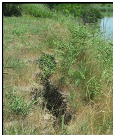
Figure 2 Lateral spreading deformations along the river embankment of Scortichino (Lo Presti et al., 2013).
