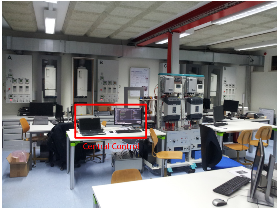
Figure B-9. GridLab laboratory general overview.
