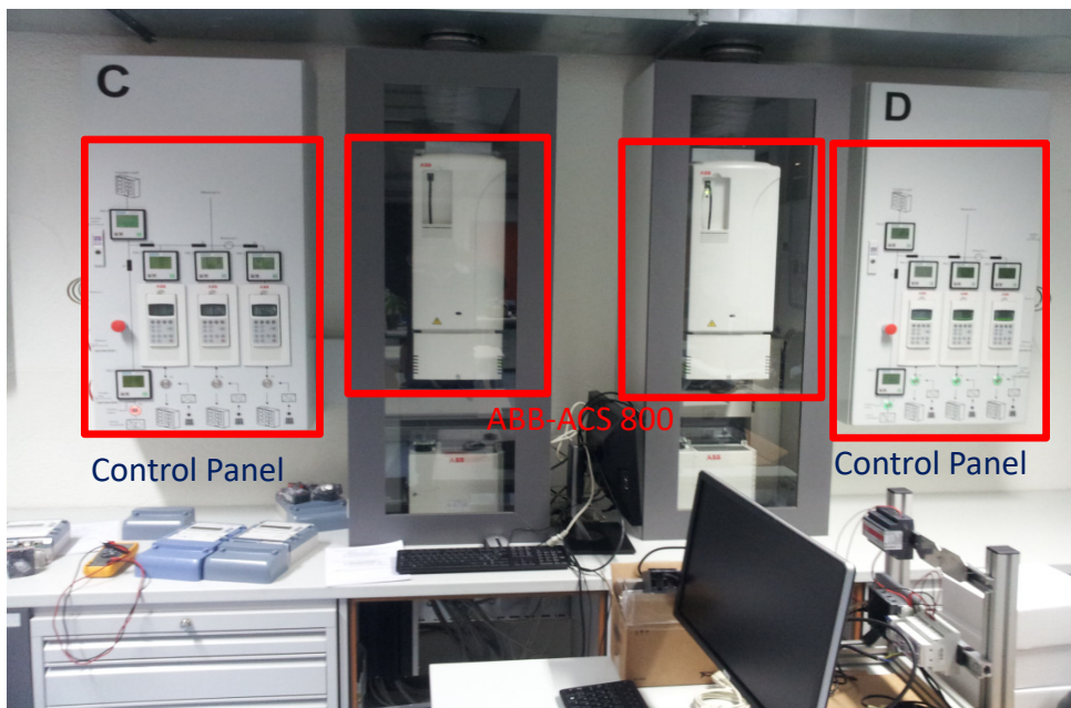
Figure B-10. GridLab laboratory: drives and local control panels.
