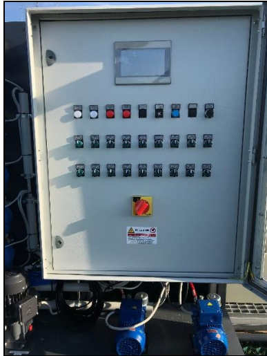
Fig. 5.9 - Check of the electrical cabinet.
