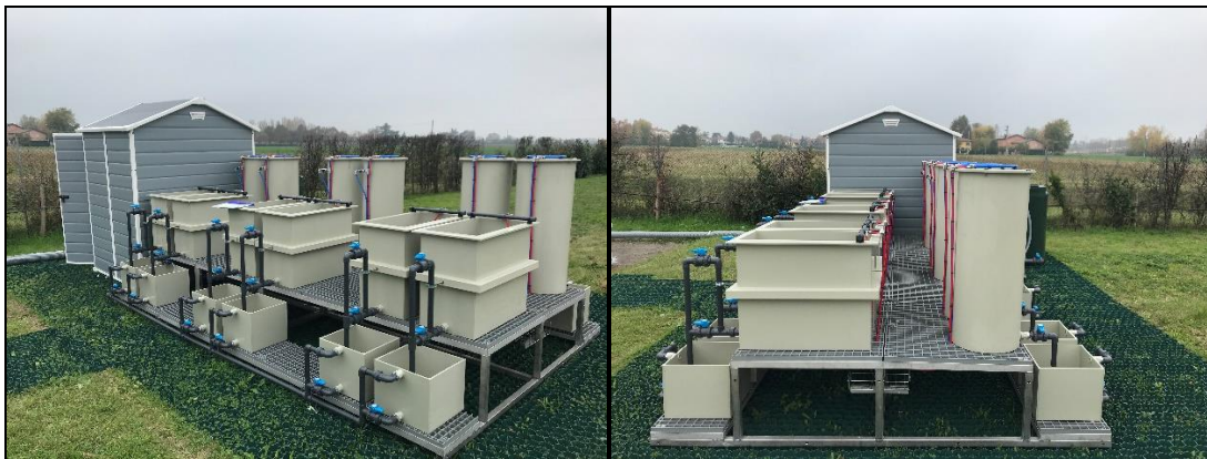
Fig. 5.2 - Installation of the pilot plant at the wastewater treatment plant of Granarolo (BO), Italy.
