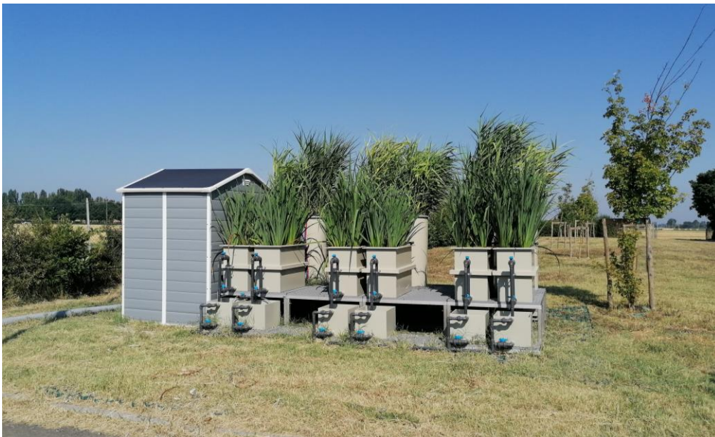
Fig. 5.10 - The constructed wetland pilot plant in operation (July 2021).
