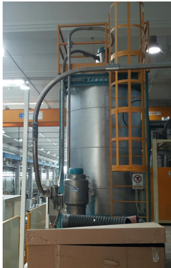
Figure 3.14 PAM002A: PET dryer on mezzanine.
