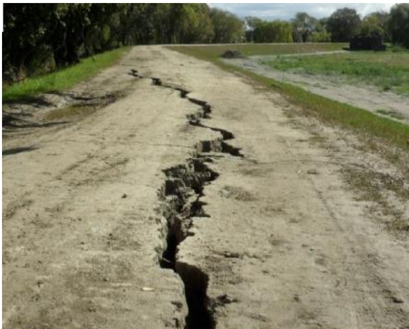
Typical longitudinal cracks on the crest of the embankment. Samples taken from sand boils proved that the surficial layer liquefied.
