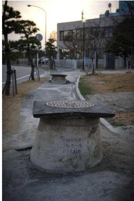
Figure 1.4 Manholes uplifting in Urayasu, Japan, during Tohoku earthquake, 11 th March 2011 (Koki Nagahama/Getty Images)
