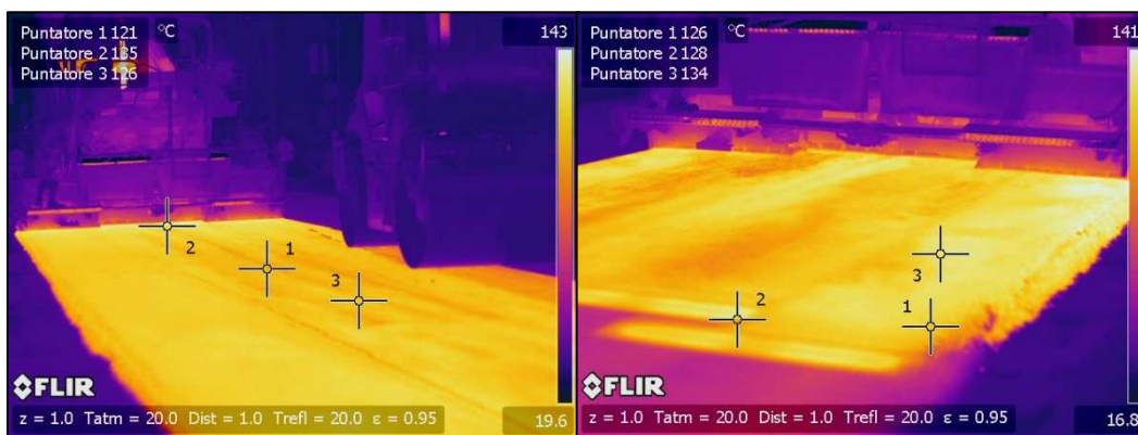
Figure 4.4: Temperature verification during laying: no rubber on the left, with rubber on the right
