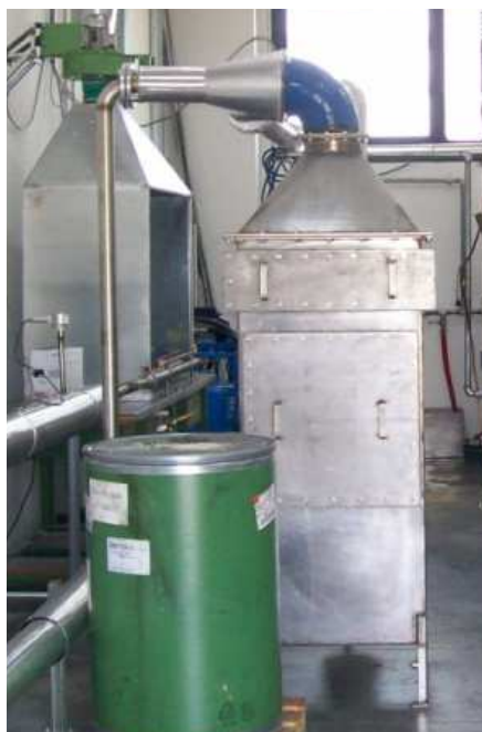
Figure 4.5 – H 2 S scrubber.
