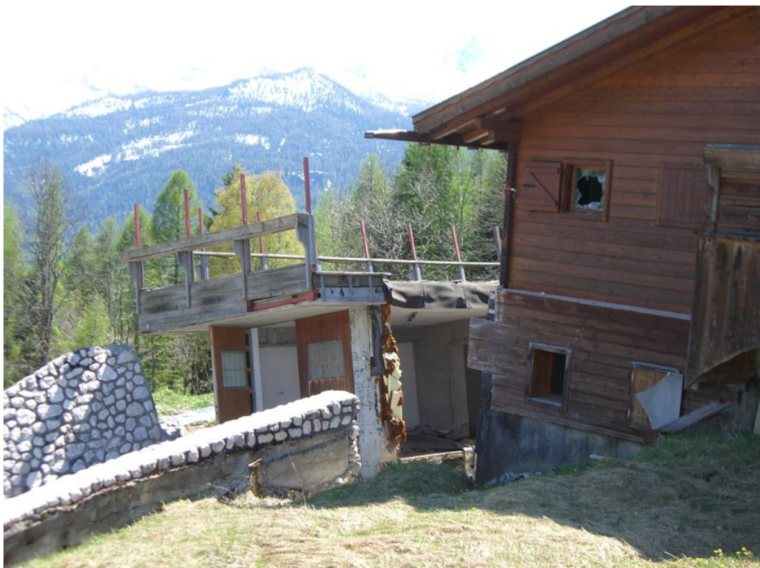
Fig. 25: a building along Sector 2 completely destroyed by the landslide moments
