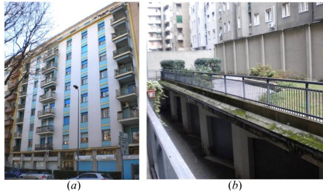
Figure 3.29. General view of the main left side façade (a) and detail of the garage zone on the right longitudinal side (b) of the building.
