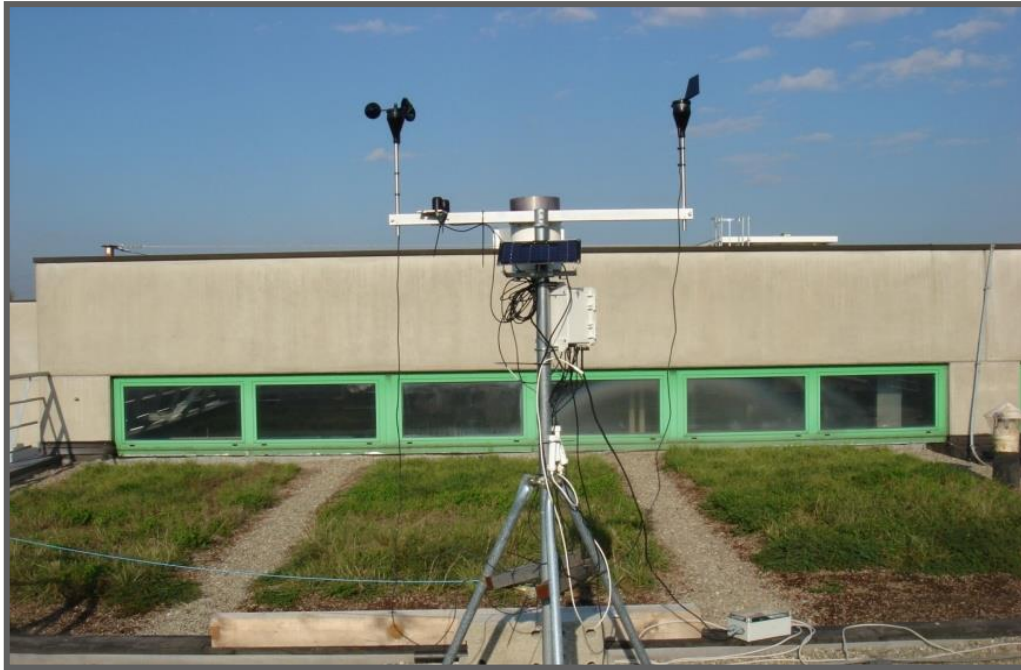
Figure 72: Installation of Green Roofs - University of Bologna Via Umberto Terracini 28 (Maglionico et al., 2014).
