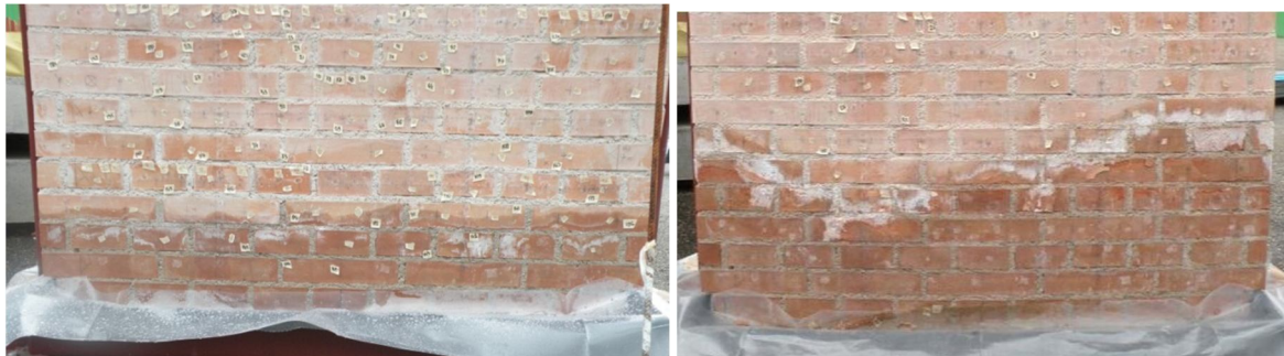
Figure 6.16: PNDE, front side, July 2010 (left) and November 2010 (right)
