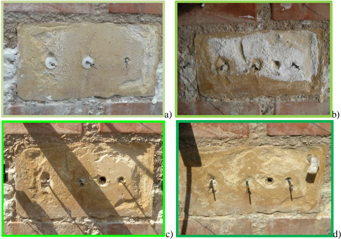
Figure 6.9: PNDB, front side, progress of deterioration in the Palestine stone: a) November 2010, b) April 2012, c) August 2012, d) September 2013
