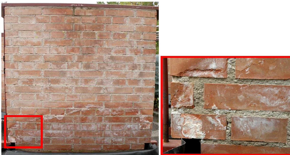
Figure 6.14: PNDD rear side, Nov. 2011, evident blistering of bricks and losses of materials on the mortar joints
