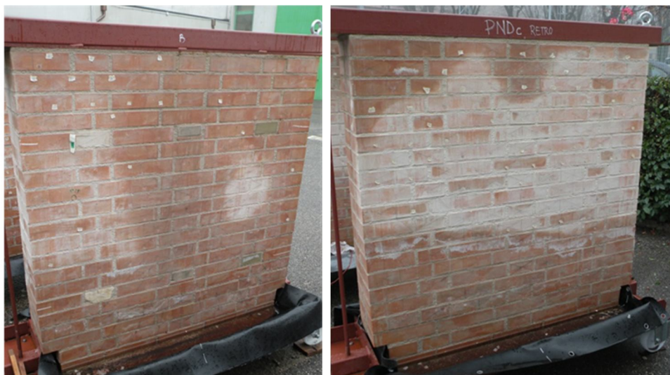
Figure 6.10: PNDA damage status of plaster on back side at the end of the second aging season (2011-11-08)
