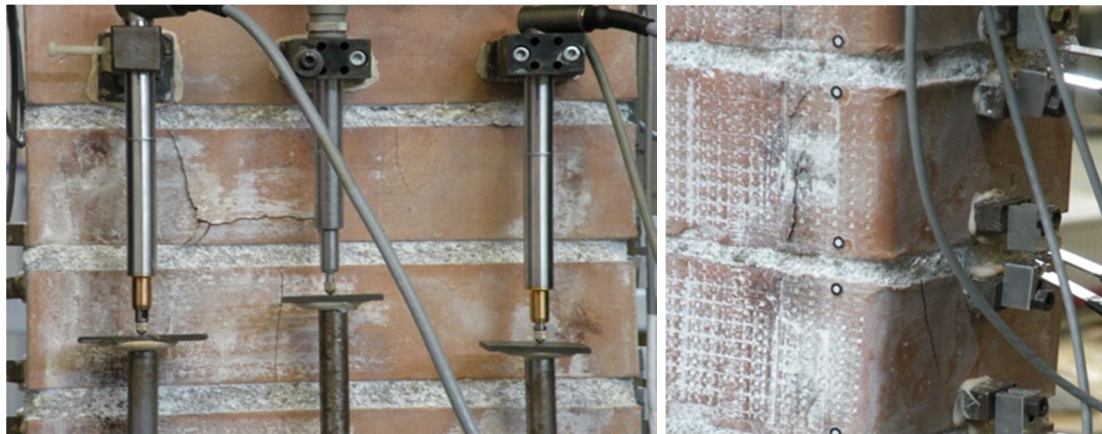
Figure 22: Six-brick column 4S1: details of the crack pattern appeared on the front (left) and rear side (right)
