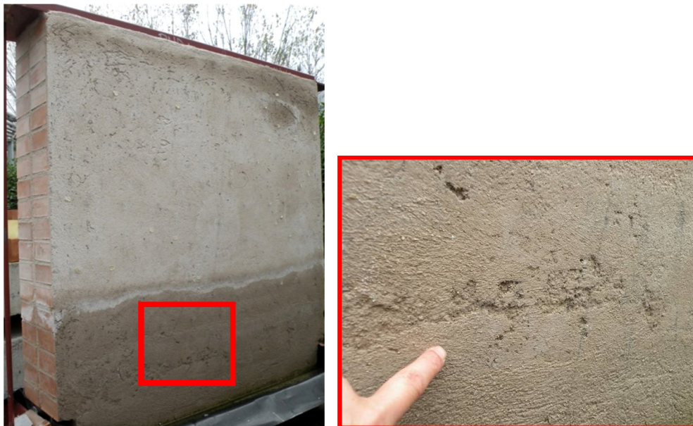
Figure 6.3: PNDA, plastered rear side at the end of the 1st ageing season (Nov. 2010)
