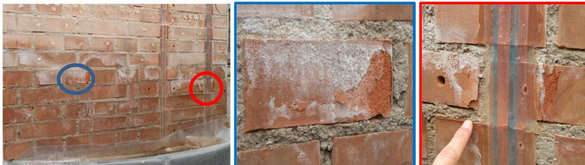
Figure 6.17: PNDE, Nov. 2010, rear side (left) and 2 brick degradation details (right)
