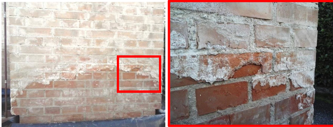
Figure 6.15: PNDD, rear side at the end of the 3 rd ageing season (November 2012)
