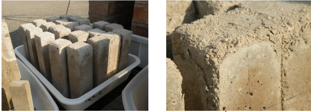
Figure 5.3: Visual decay on mortar prisms during the 3 rd ageing season. Sodium chloride contamination: general view (left) and detail (right)
