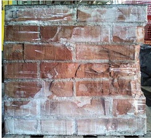
Figure 8.33: Wallet II: exfoliations and cracks visible at ...kN (left); crack pattern at the end of the mechanical test (right)
