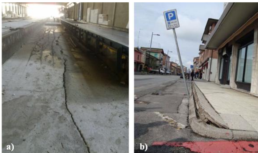
Figure 3.2: a) Ground fractures and associated sand ejection observed at Mirabello industrial area after the 20 th May earthquake; b) damages in the centre of the village (Courtesy of Prof. G. Vannucchi, University of Florence, Italy)
