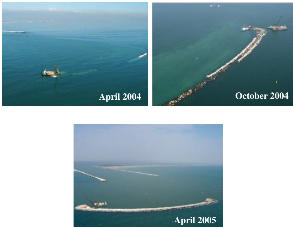
Figure 7.24: Construction history of the breakwater in the Chioggia Inlet (images taken from the website salve.it )
