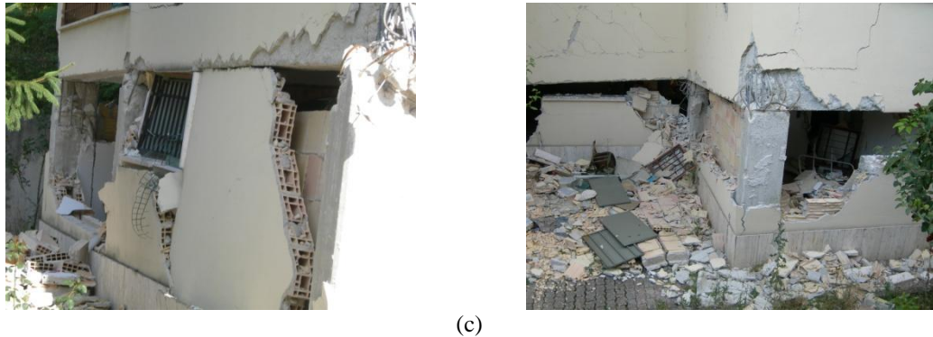
Figure 3.4: Damages observed for the studied building. (a) Soft/weak story mechanism; (b) Shear failure in columns; (c) Infills failure.
