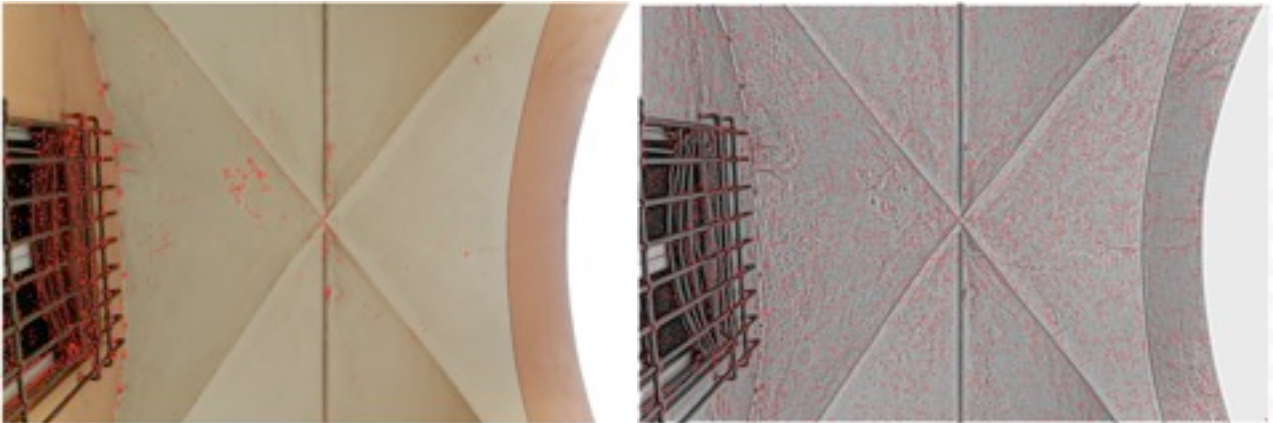
Figure 2.29 Detected features on photo of vault. Left: colorful image. Right: Wallis-filtered image
