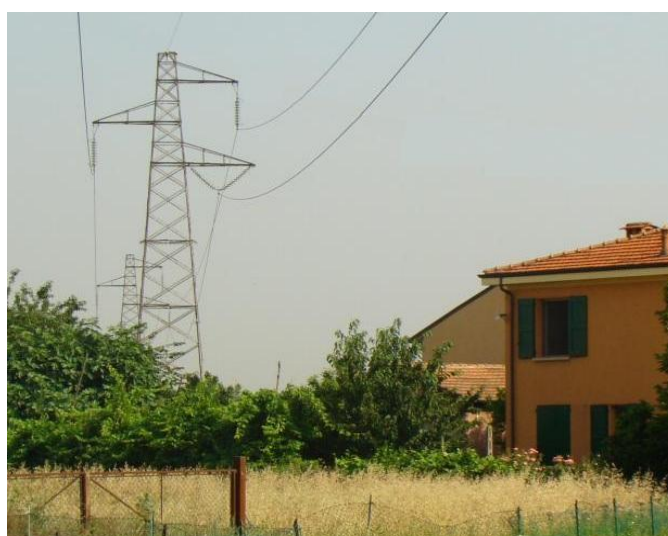
Figure 6.15: Photo of the single-circuit power line close to the measurement point.
