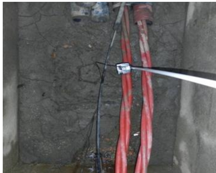
Figure 3.12: Photo of the twisted double-circuit power line inside the inspection well, along with the magnetic field measuring probe (the black cable is a signal cable and does not affect the measurements).
