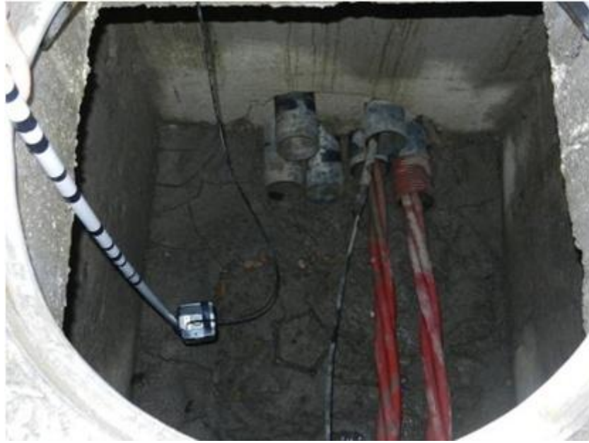
Figure 3.16: Photo of the probe at 0.57 m left from cable 2 having positioned the cane at the other end of the well opening.
