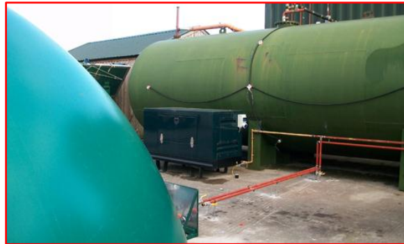
Fig. 2.45: High pressure tank of biogas (as cited in ZORG, 2012)
