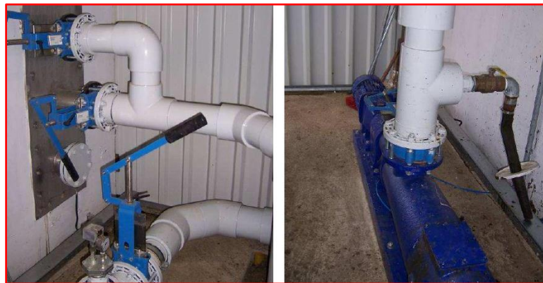
Fig. 2.19: Stop-valves (left) and pumping system (right) (as cited in Rutz, 2006 cited in Al Seadi et al. , 2008)
