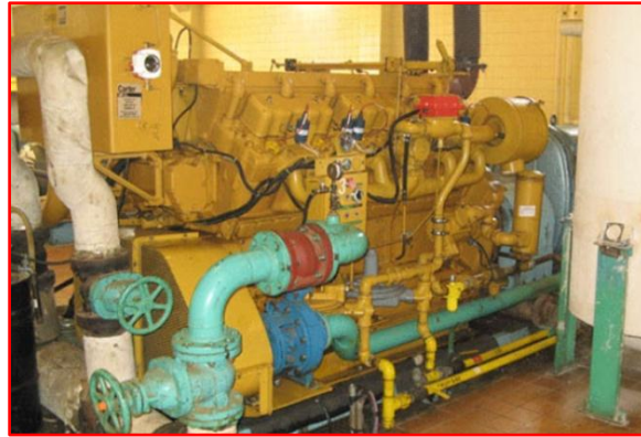
Fig. 2.54: CHP unit equipped with pilot Injection gas engine
