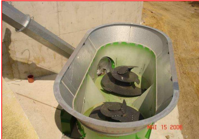
Fig. 2.24: Feeding container equipped with screw conveyor, mixing and crushing tools (as cited in Agrinz, 2006 cited in Al Seadi et al. , 2008)
