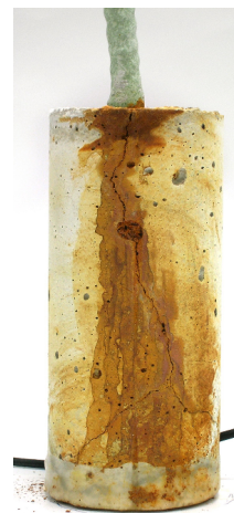
Fig. 39: Corrosion evidences (top and lateral surfaces) on M-LLSFA 2.0-21 (a), M-HLSFA 2.0-21 (b), M-CEMII-21 (c)
