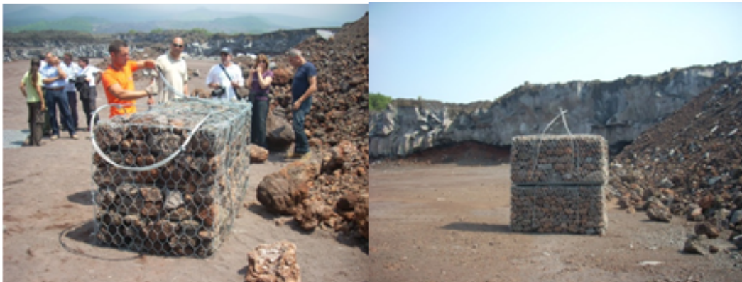
Figure 4.8: Experimental test: filling of the gabions stacked on top of each other.
