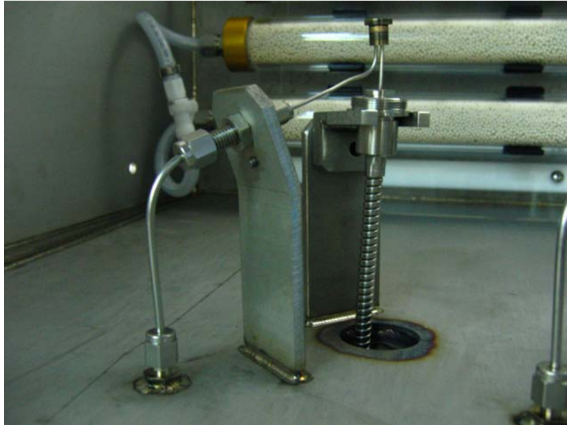
Figure 6-12 - Particular of the connection between the feeding pipe and the sensor capillar
