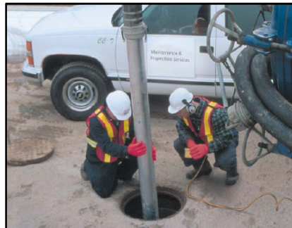
Figure 3.2 - Maintenance operations of a hydrodynamic separator
