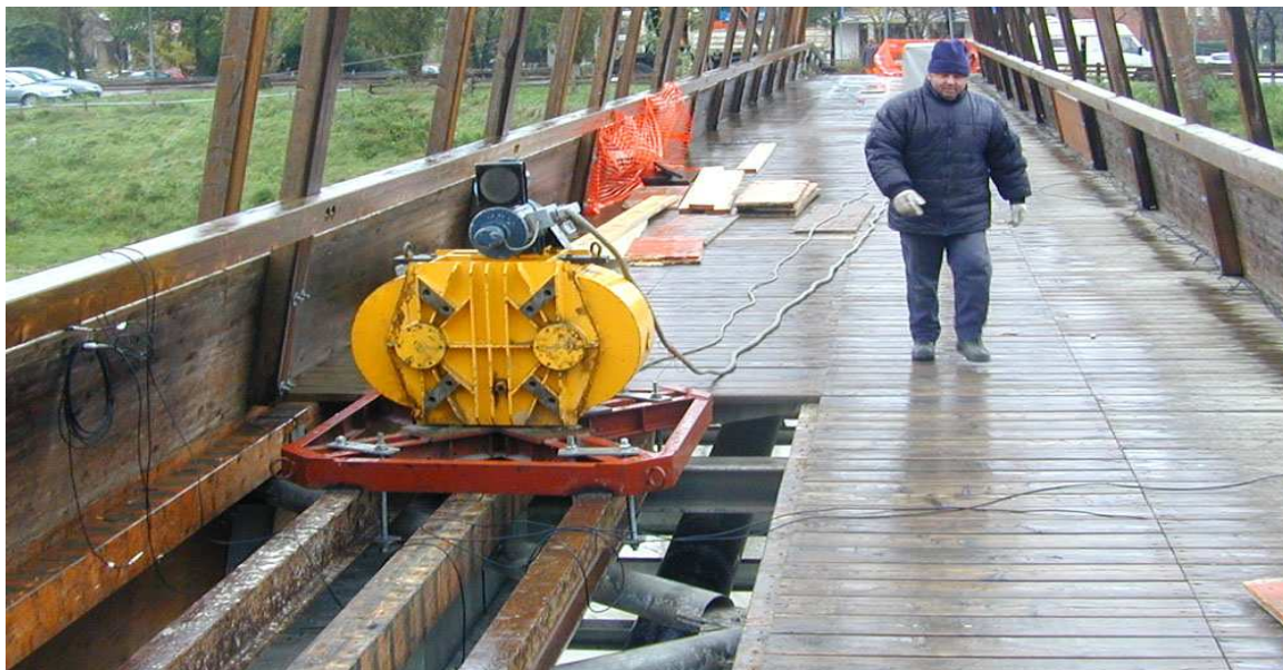
Figure 2.5.3 The electromechanical shaker
