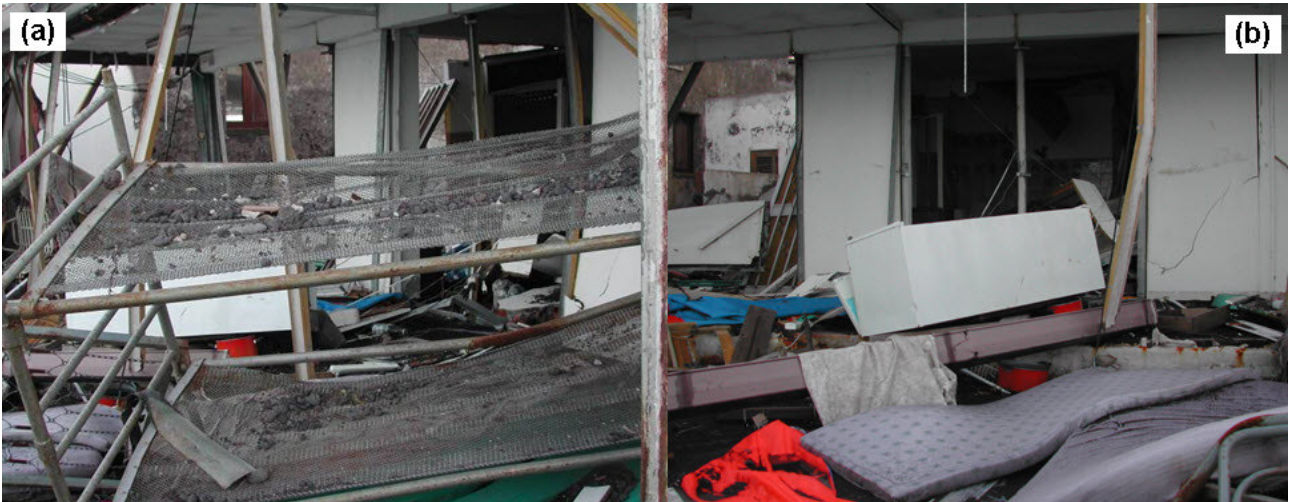
Figure 12. Two pictures of building #5 (Punta Lena, Stromboli – Figure 6) taken after the 2002 tsunami. The flow broke doors and windows down, penetrated indoors and dragged the building contents outside (Figure 12a). A large crack can be observed in the front side wall (Figure 12b). However, that wall does not appear to be part of the load-bearing structure of the building, as does the undamaged column at its right. The PTVA-3 Model classified building #5 as having an “average” RVI score.
