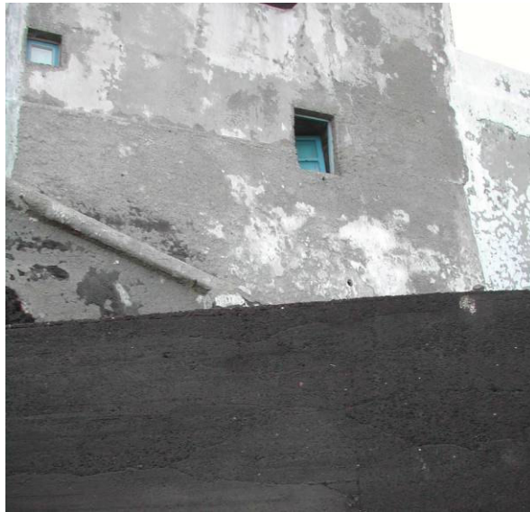
Figure 8. View from north-west of building #1, at Piscità (Stromboli – Figure 4). The picture was taken a few days after the 2002 tsunami. The only visible damage is an unhinged window at first floor. The PTVA-3 Model classified building #1 as having a “very low” RVI score which correlates well with the actual damage sustained by this building.
