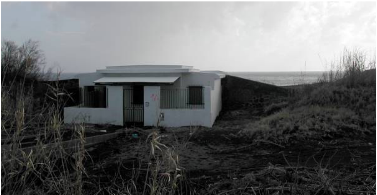
Figure 13. View of the eastern side of building #6. The picture was taken few days after the 2002 tsunami. Building #6 is a Coastguard station on the beach of Scari (Stromboli – Figure 6). As clearly shown by the picture, the seaward side of the building is totally “covered” by a coastal dune. The PTVA-3 Model attributed to building #6 an “average” RVI score.
