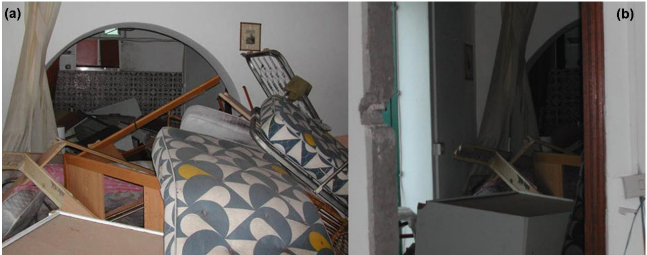
Figure 10. Two pictures of building #3 (Punta Lena, Stromboli –Figure 6) taken after the 2002 tsunami. Figure 10 (a) shows damage to interiors. Figure 10 (b) a view of the main entrance of the building, where the door have been ripped off the wall. The PTVA-3 Model assigned to building #3 an “average” RVI score.
