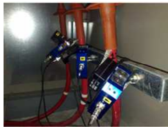
FIGURE 3.1 HFCT sensors installed inside the switchgear, around the cables ground lead.
