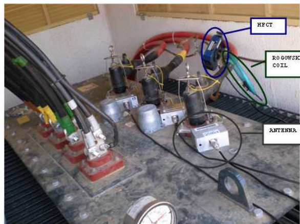
FIGURE 4.8 On-line PD measurement setup for a 400V / 15 kV oil insulated transformer in a solar park. PD detection carried out through HFCT and Horn Antennas.
