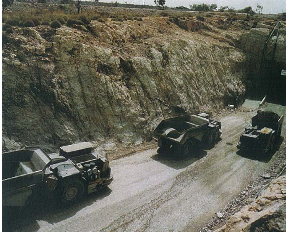
Dumper Atlas Copco MT5000 all'imbocco della miniera Pillara – Western Metals Lennard Shelf Operations – Western Australia
