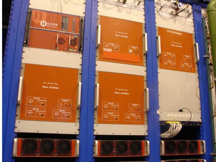
Figure 2.20: One of the four ALICE TOF rack low-voltage subsystems with the SY1527 mainframe, the A1395-Service and three A1395A-Power power supplies.
