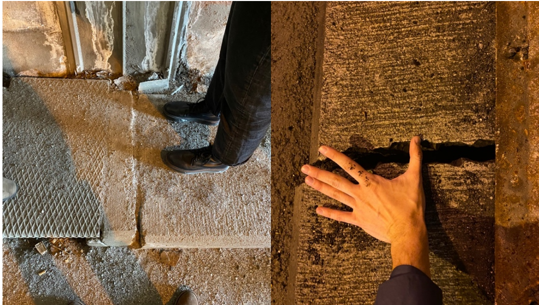
Figure 23 - Photographs of the resulting gap in sidewalks in different adjacent segment connection points
