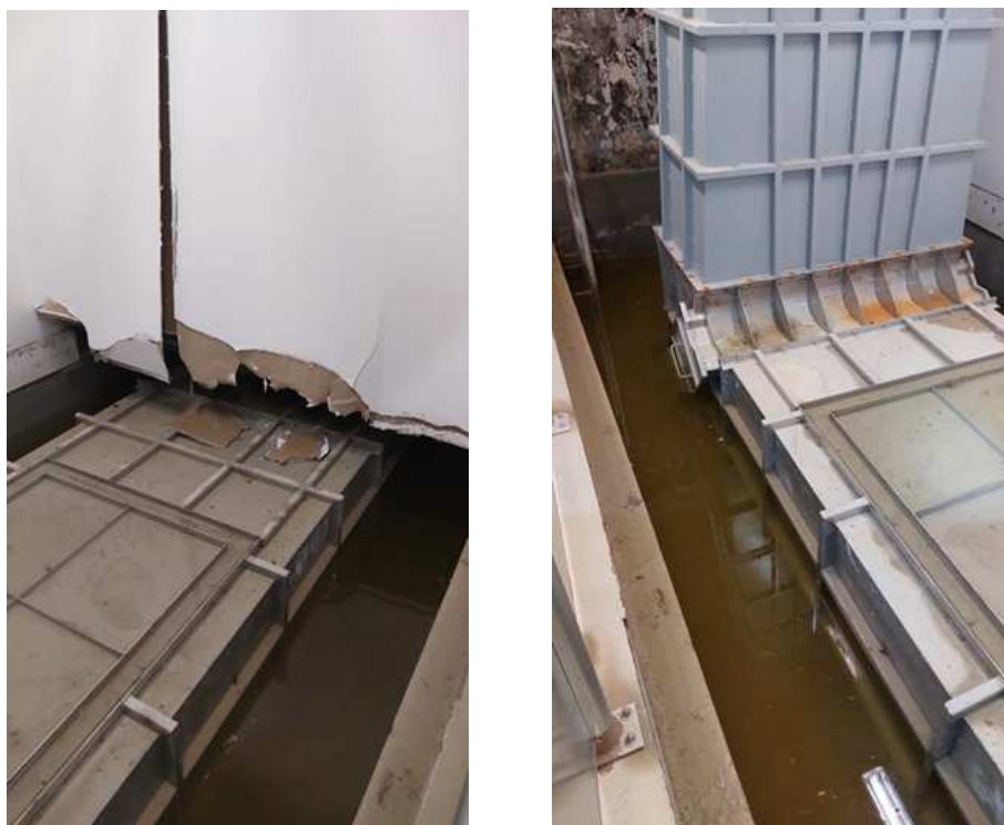
Fig. B.15 damage to plasterboard and flooding of the lower cavity housing part of the wind tunnel return circuit.
