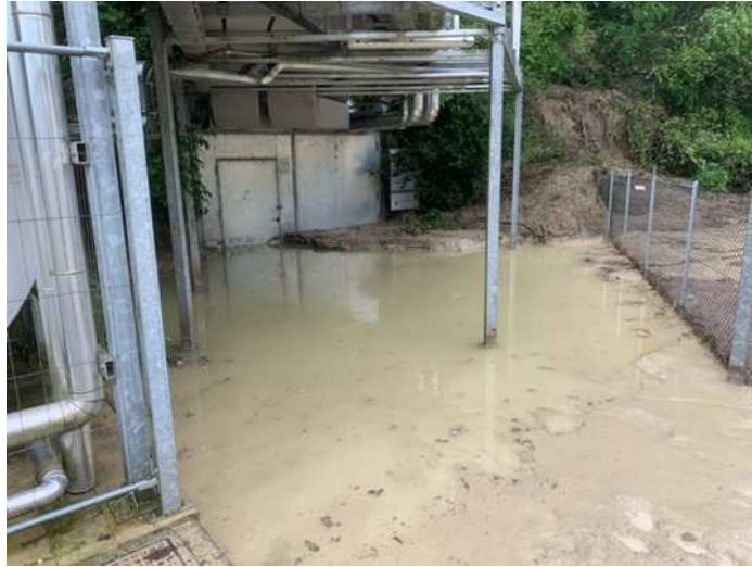
Fig. B.10 Flooding near the main entrance.
