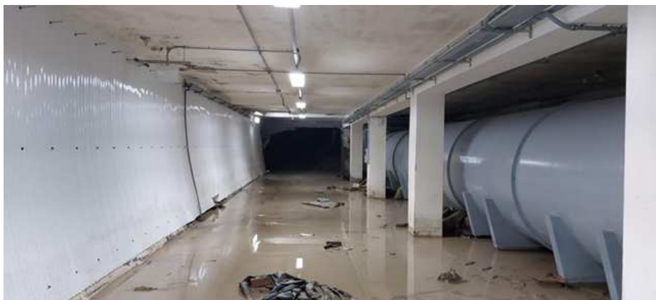
Fig. B.13 State of the laboratory at first entrance following the flood of 16 May.
