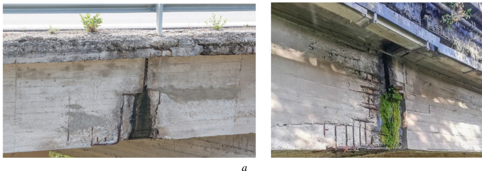
Figure 4.3: Example of deteriorated Gerber saddles in RC road bridges
