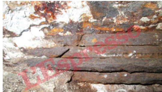
(b) Corroded strands
