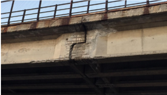
(a) Damaged Gerber saddle
