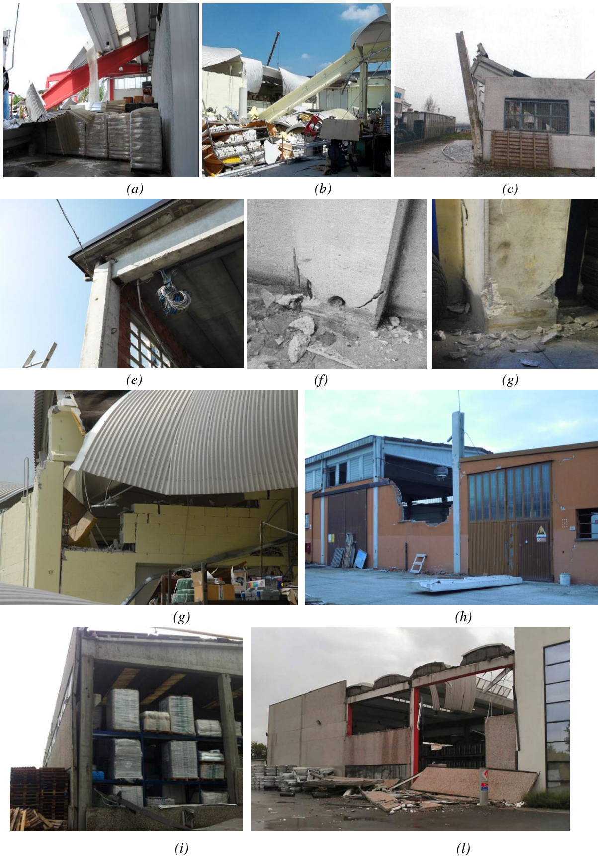
Figure 19. Collapse and damage mechanisms observed in the buildings in the case-study area of San Felice.
