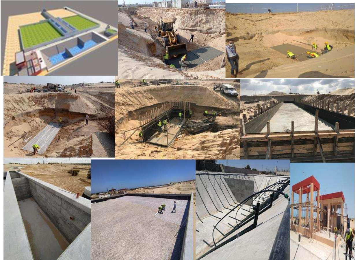
Fig.4- 14_ General pictures of the main construction phases of the plant in real scale. (Photo credit: Authors)
