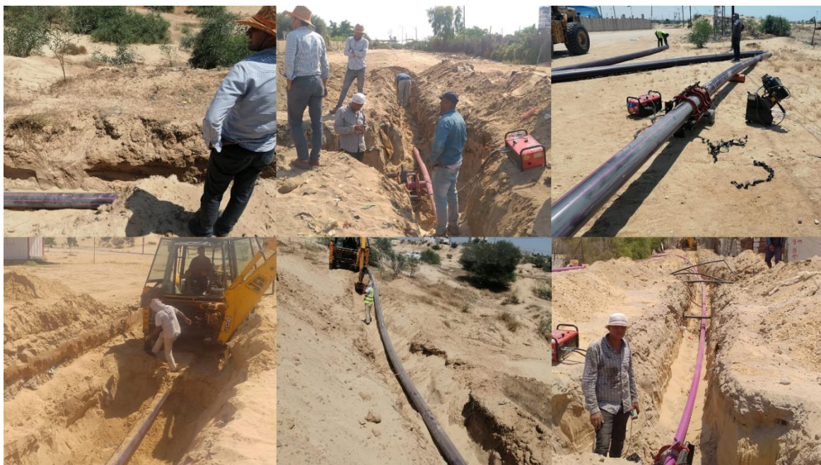
Fig.4- 17_ Pictures showing the main construction phases of the irrigation network. (Photo credit: Authors)
