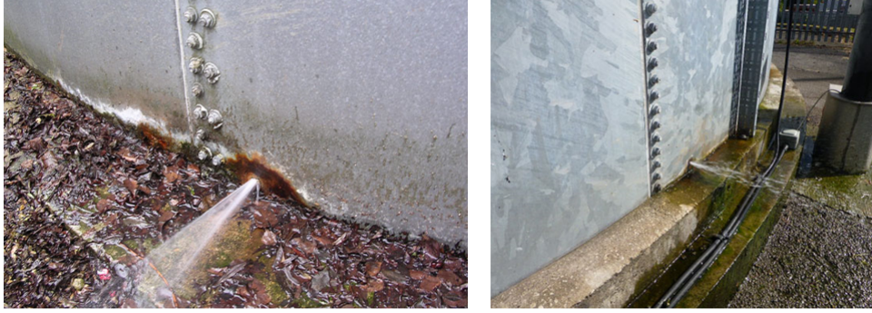
Figure 2: Active leaks at the AST wall due to corrosive perforations, Generis (2019).
