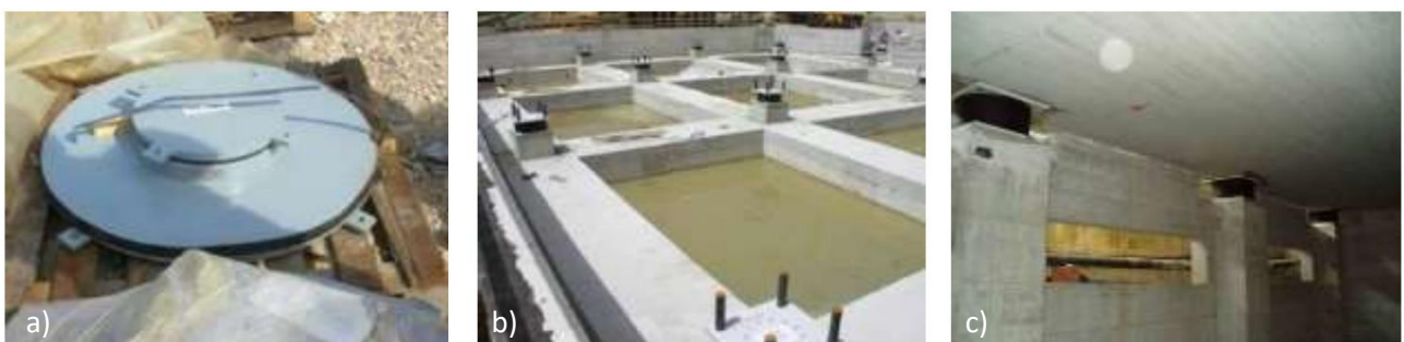
Figure 23 – Examples of isolator applications. A) One of the 12 isolators applied in the new school Francesco Jovine in San Giuliano di Puglia; b) some of the 61 high damping rubber bearing (HDRB) isolators installed at the base on the above-mentioned school; c) some of the 16 HDRB installed on an isolated floor of a building in Foligno (Perugia) – Source: [60]
