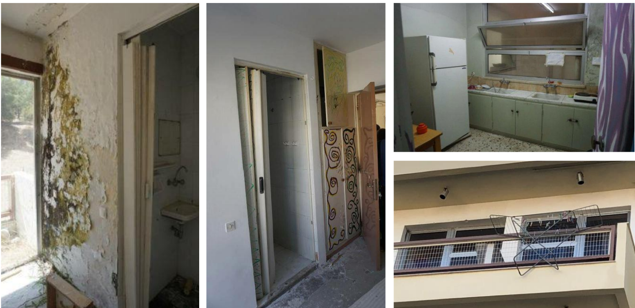
Figure 288 – Photos of the Athens case study showing the current situation of degradation and lack of space
