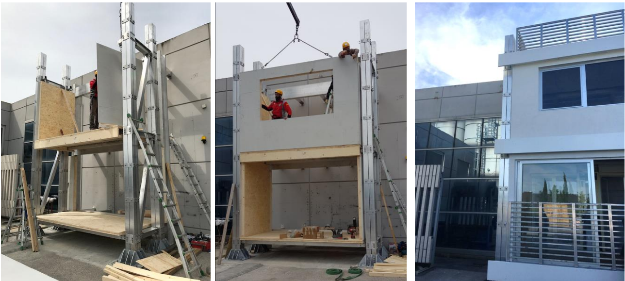
Figure 295 – Photos during and on completion of the mock-up of Pro-GET-onE in the ALIVA Srl plant – Source: [211]
