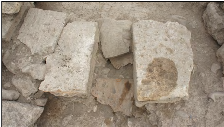
Fig. 2.48 - The channel D.4589 through the southern wall W.4584 with remains of a metal plate. From south.
