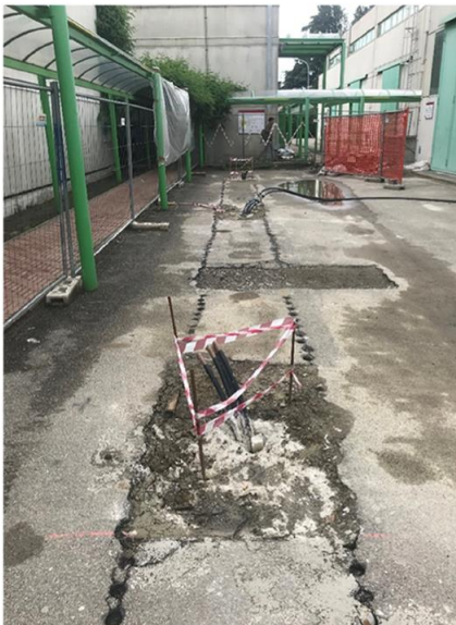
Figure 2.20 – View of the top of the borehole heat exchanges installed outside the laboratory.
