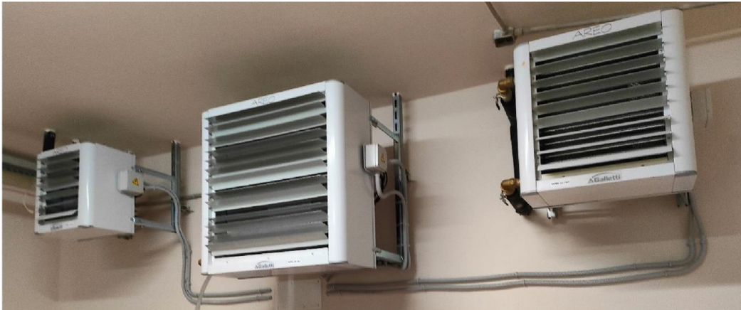
Figure 2.19 – View of the test three air -heaters placed inside the climatic chamber.
