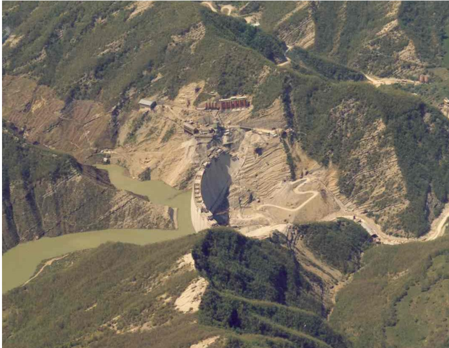
Figure 1.1. Aerial view of Ridracoli Dam during construction work (courtesy of Romagna Acque – Società delle Fonti S.p.A.)
